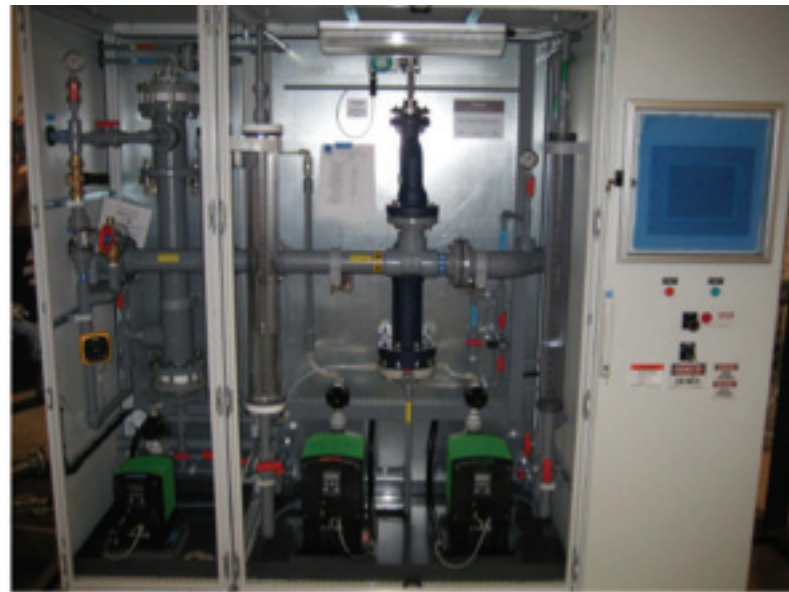
Figure 1 -PURATE SVP Pure chlorine dioxide generator (SVP-Pure \text{ClO}_2 Generator (MSA)).
